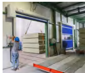
Explosion-proof door of paint shop
